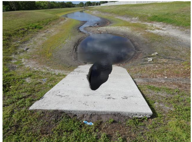
Stormwater Drainage Mitered End Section
